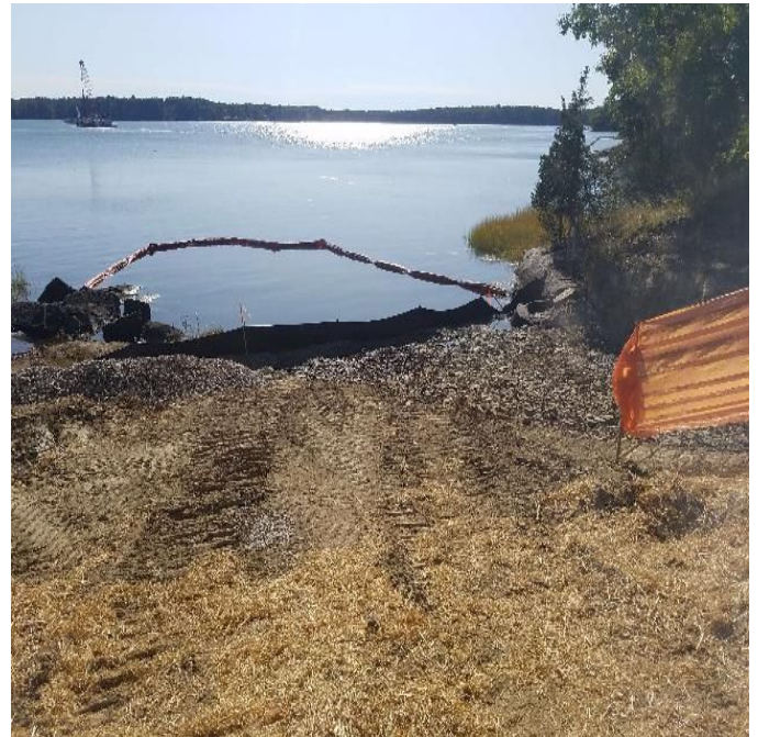
Fig 10: Erosion controls installed downslope of Blu Rock's trenching activities on the west side of the Bay. Viewing east. (9-24-19).
