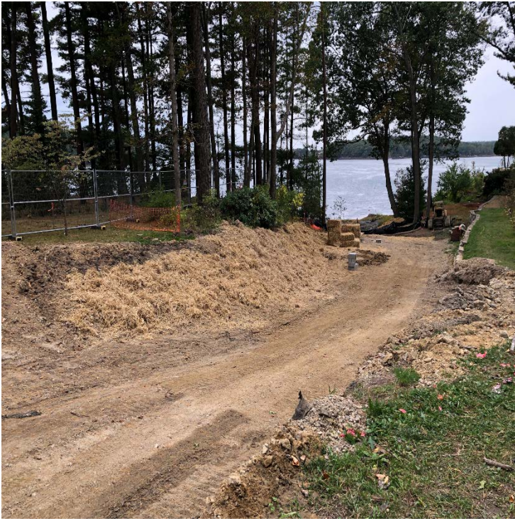
Fig 17: Straw placed on slope of the access to man hole- Newington side of Bay. Viewing west. (9-25-19).
